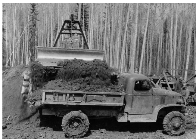
Figure 3: Dozer drifting loose soil into a 1940 Chevrolet 4x4 1-1/2 ton (1360 kg) capacity dump truck. It is hauling fill for an airport access road in May 1942 (Source: US NARA).
